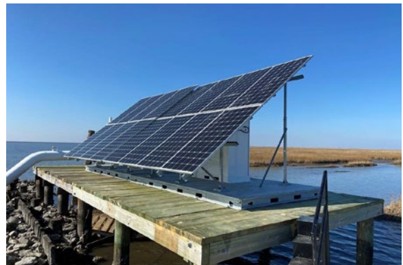
▲ Coastal pipeline platform using CPX Cathodic Controller and solar power.
